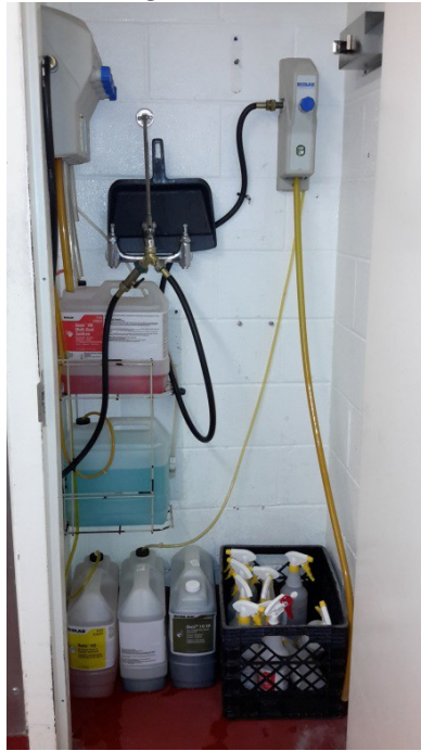
Janitor Closet- Cleaning solutions- 21 lbs., from floor to 40"
