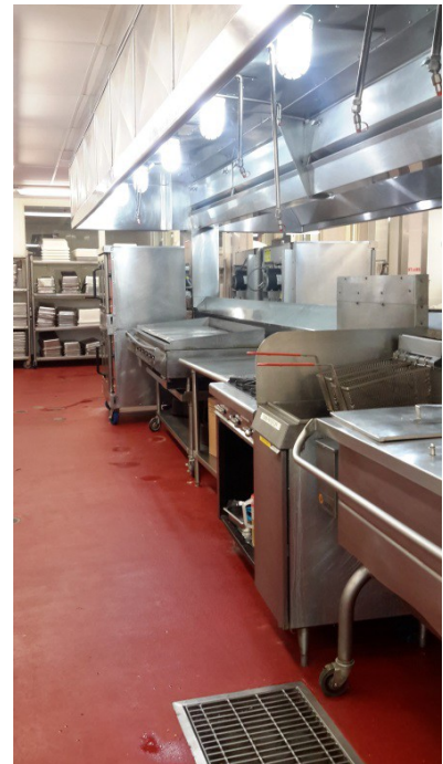
Deep Fryer, Stove Top, Grill, Ovens
